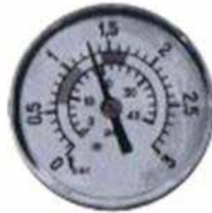
1.3kg/cm 2 -18.5PSI: In pressure Need to backwash
